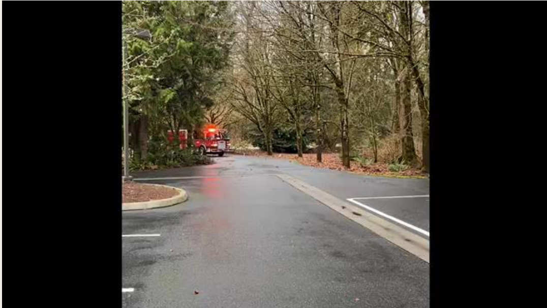
OPEN TRENCH WITH A LINE FRACTURE
